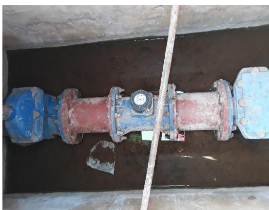
Figure 15: Bulk meter installed by STWP on rising mains to reservoir in Chiredzi town. Improves measurement of water entering the system (system input volume), which is a key input for NRW calculations.
