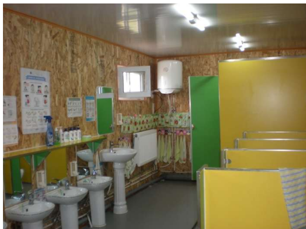
Inside indoor WASH container van in Burentogtokh kindergarten
