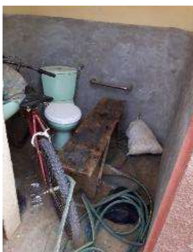
Photo 18: Public sanitation facility in Ulongue: cabin for people with disabilities used as warehouse
