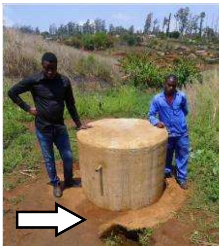
Photo 11: Damaged water catchment in Espungabera
