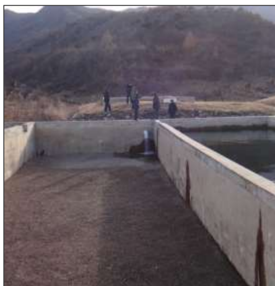
Incorrect SSF Operation, Unchon County
