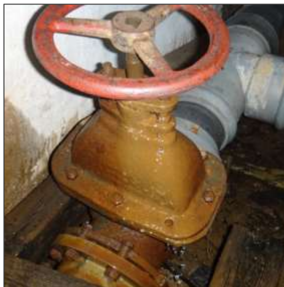
Failing Valve, Yontan County (see Section 4.5)
