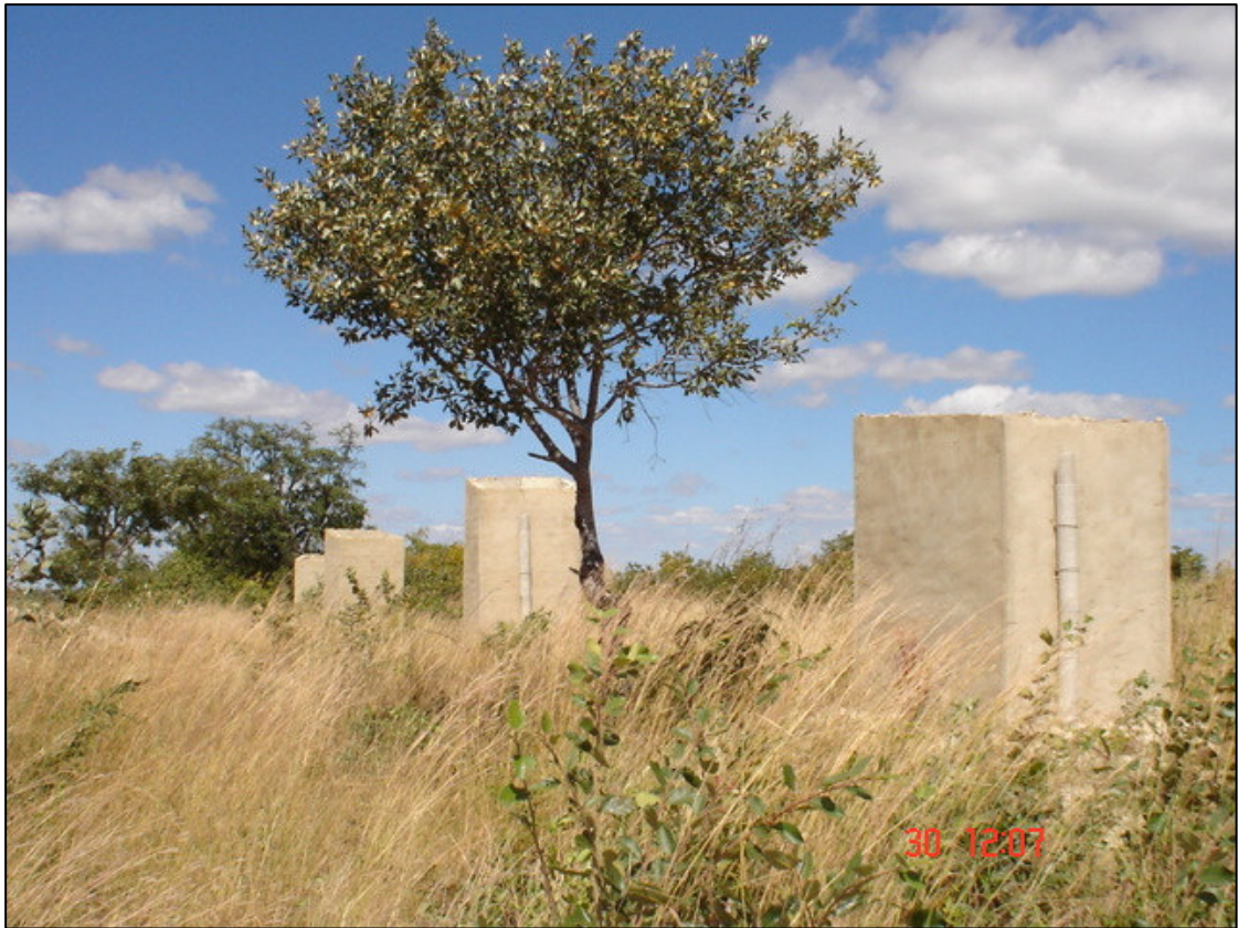
Photo 3: Constructed toilets yet to be roofed at Chalimongela Basic School in Kalomo District
