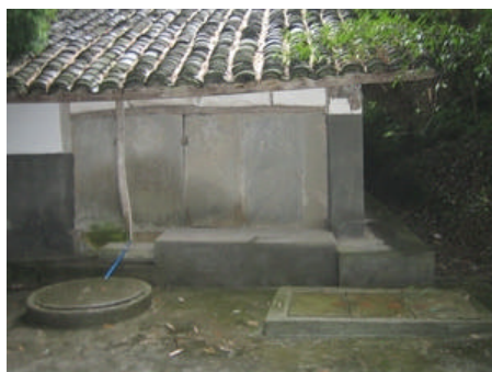
A bio-gas plant in a rural household treating human excreta and pig manure that generates clean energy for family cooking and lighting
