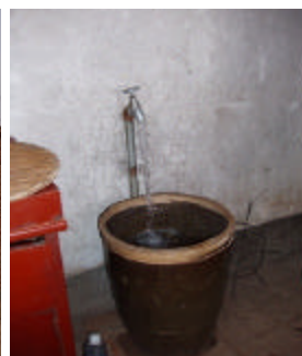
Piped safe water is distributed to all rural houses in the resettlement colony
