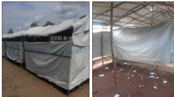
Pictures 5 and 6: School with tarpaulins provided by UNICEF in Kananga, with signs of deterioration
