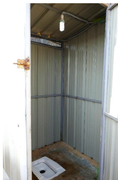
Figure 5: Light installed inside a latrine in an informal settlement
