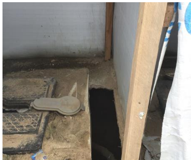
Figure 4: Emergency latrine in Zamai, Mayo-Tsanaga, Far-North Region
