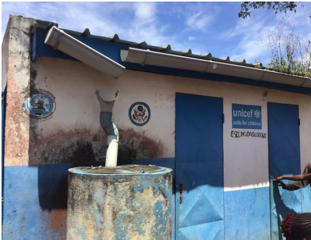
Figure 2: Broken rainwater harvesting system at a school
